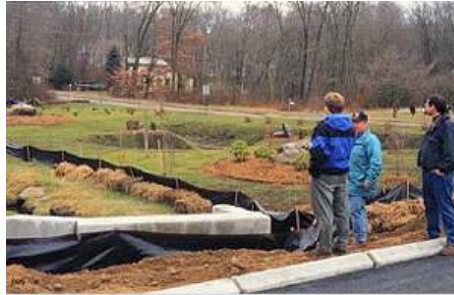
Construction reviewers periodically inspect construction sites to ensure that contractors have installed and maintained their erosion and sediment controls properly (Source: University of Connecticut Cooperative Extension System, 2000)
