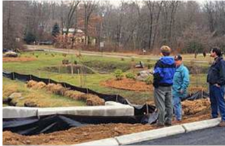
Construction reviewers periodically inspect construction sites to ensure that contractors have installed and maintained their erosion and sediment controls properly (Source: University of Connecticut Cooperative Extension System, 2000)
